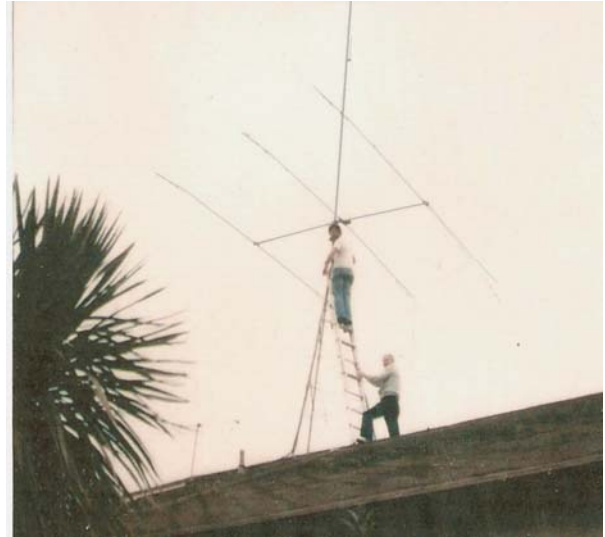
W1ZE (then WA6MUP) & Ed Reinburg, W6JI installing HF Yagi and 2-meter J-Pole March 1977
